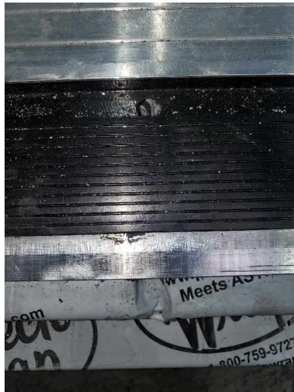
Photo No. 14 Sill Drainage
