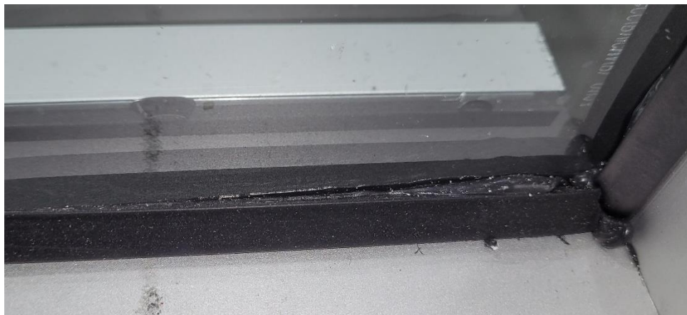
Photo No. 9 Interior glazing gasket with silicone at corners
